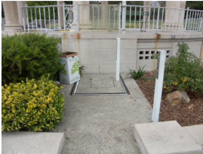
Existing non-functional underground lift. The City is currently responding to a lawsuit relating to this lack of accessibility.
