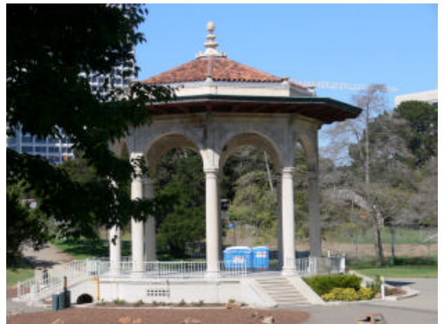
View from SE. Portable toilets are brought in for special occasions. South stair has a handrail; the other stairs have no
