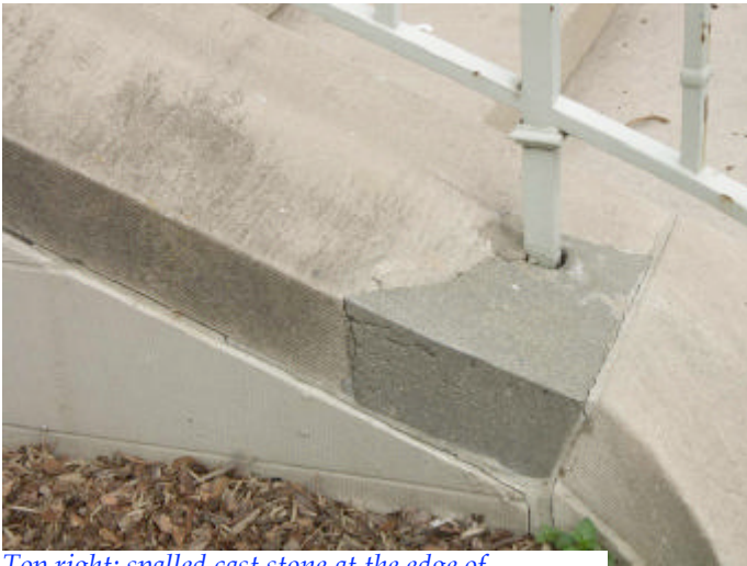
Top right: spalled cast stone at the edge of bandstand floor. Rusted round pins may be from a previous repair.
