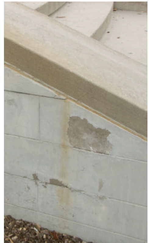
Painted cast-stone wall. The original material is exposed where paint is chipping off. Cast-stone stairway is unpainted.
